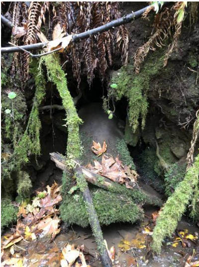
A failed culvert at Fort Hoskins to replace
